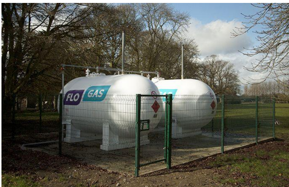
Boilerhouse was temporarily supplied with LPG while the contractor (Kingmek Limited) organised to have natural gas on site. This demonstrates the capability & diversity of the De Dietrich boilers with an adjustment of the gas valve allowing the boilers to be fired on LPG and then converted to natural gas once supply was available.
