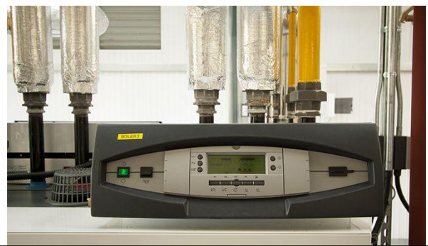
DeDietrich Diematic M3 master panel supplied with the ECO 230 Master boiler allowing control of all 6 boilers on site through one panel. The De Dietrich Eco boilers are supplied with all water and gas connections made from the boiler top, allowing for boiler back to back positioning. The Dietrich panel is interchangeable i.e. side or front facing
