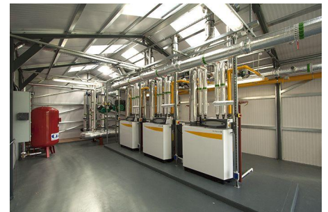
Plantroom detailing the De Dietrich ECO C230 Boilers in Cascade c/w Jeremias Flues and Wilo Circulators.
